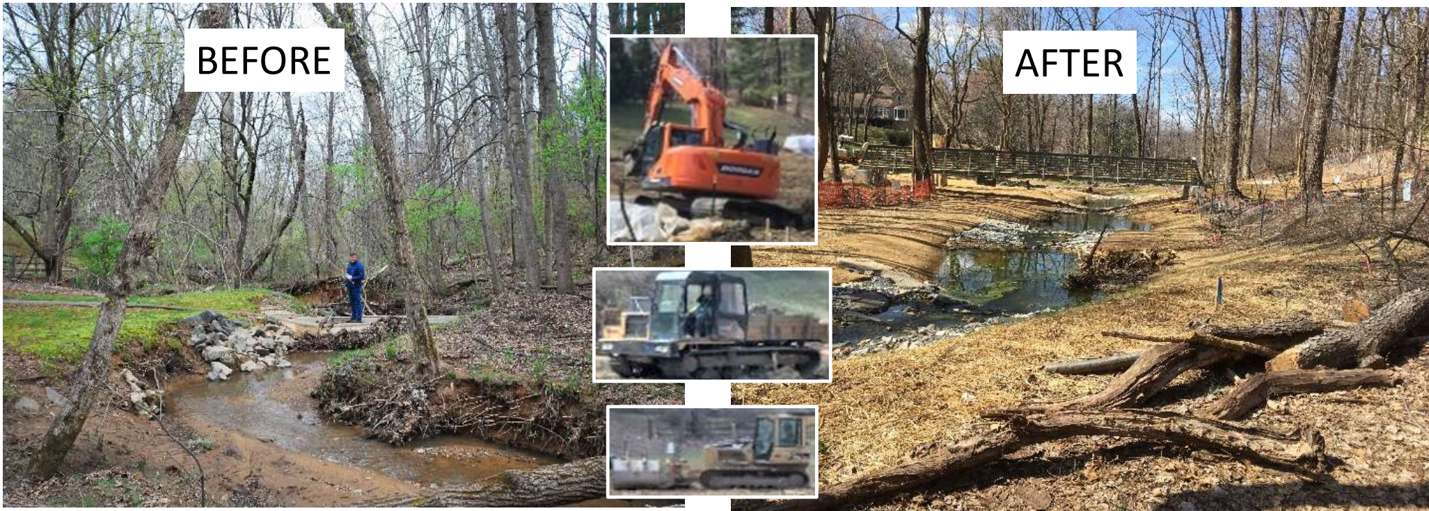
Before Montgomery County DEP “stream restoration” on Falls Reach. (Photo by DEP)
